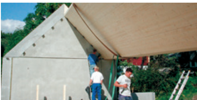
The installation of large laminated timber elements requires tremendous precision and accuracy.
