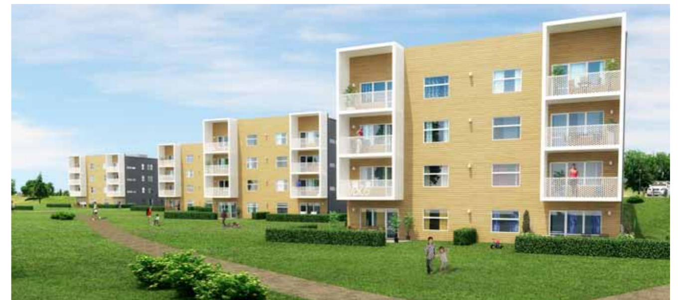
Four-storey Modular dwellings with 2-5 room units are being erected at Barkarby Hage outside Stockholm, supplied by Moelven ByggModul AB.
