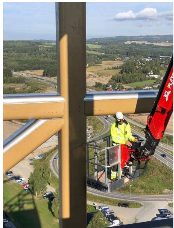
Figure 7 Glulam sections throughout the pergola have rounded edges to reduce the wind load
