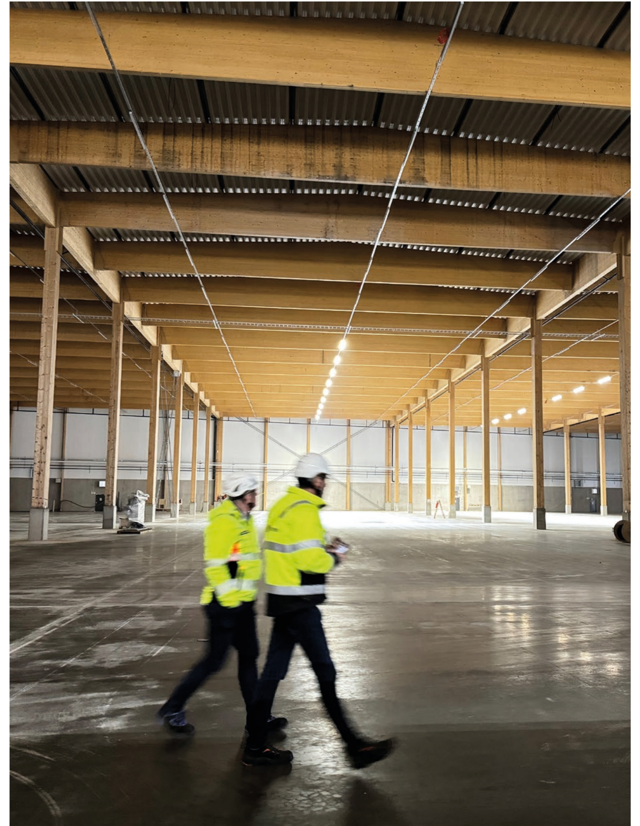
Elgiganten's new warehouse and logistics facility in Jönköping will be one of the largest in the Nordic region. The load bearing structure of the 86,000 square meter building consists entirely of glulam from Moelven Töreboda AB and Moelven Limtre AS. A total of 6,300 m 3 of glulam was supplied by Moelven. The glulam binds biogenic carbon corresponding to approximately 4,400 tCO 2 e. By comparison, the UN has calculated that the average carbon footprint per capita in Norway and Sweden in 2020 was approximately ca. 6.7 tCO 2 e and 3.2 tCO 2 e respectively.
